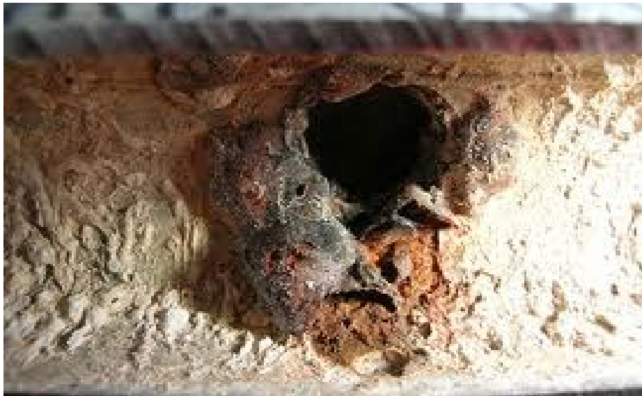
Figure 5: Damage caused by the presence of microbes
